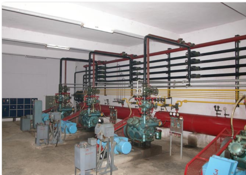
A cold store plant room with Kirloskar NH3 compressors
