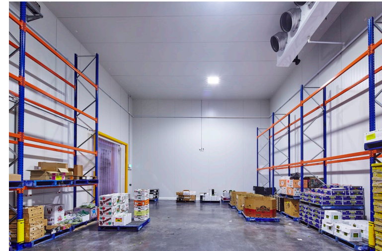
Source: Rainfresh Cold Store VIC, ASKIN Performance Panels
